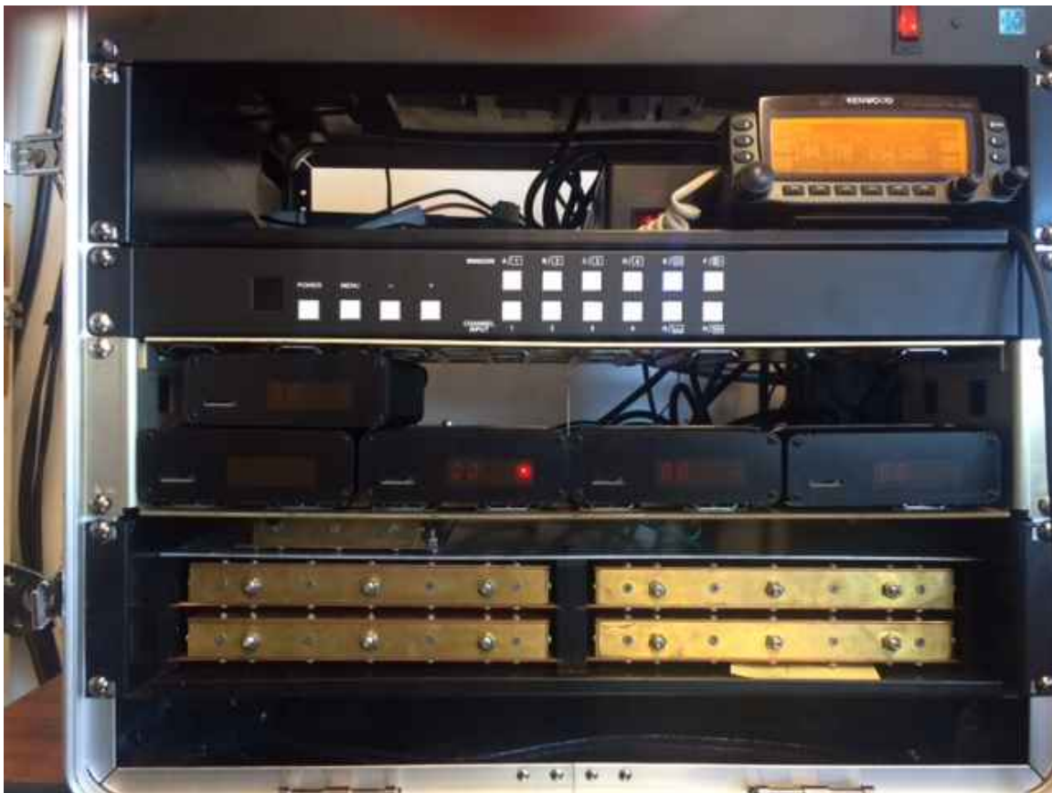
Fig. 3 Close up of the front of the new Quad DVB-T Receiver. Key items seen top to bottom are the 2m FM transceiver, the HDMI quad processor, 4 Hi-Des DVB-T receivers, and 4 Spectrum International band-pass, channel filters.
